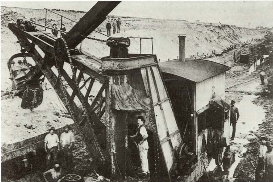
Where larger quantities of earth were to be excavated, as in the construction of the Coope canal at Fisherman's Bend in Victoria, the use of a steam navy became practicable.
